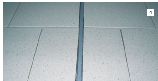
4 REMEMBER TO INSTALL PERIMETER JOINTS AND BLANKE EXPANSION JOINTS PER TCNA GUIDELINES EJ171.**
